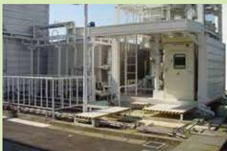
Waste water regenerating system
